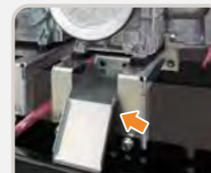
Membrane Panel Visualization of leakage from pumping unit
